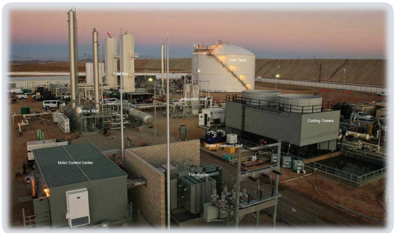
Figure 10: Clean Energy’s Boron, CA 160,000 gallon per day LNG Plant. (Photo Courtesy of WESPAC Energy)
